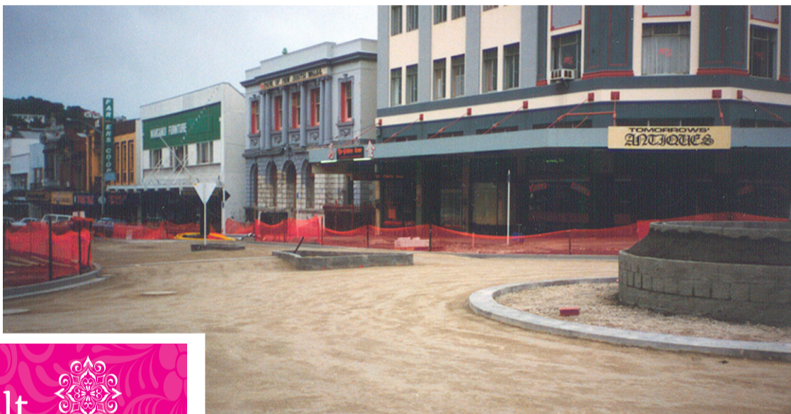
The fountain installation, pedestrian crossings and gardens being installed in the bridge block area.
