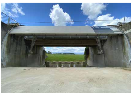
Looking through one of the open Moutoa floodgates during a dry spell in December.
